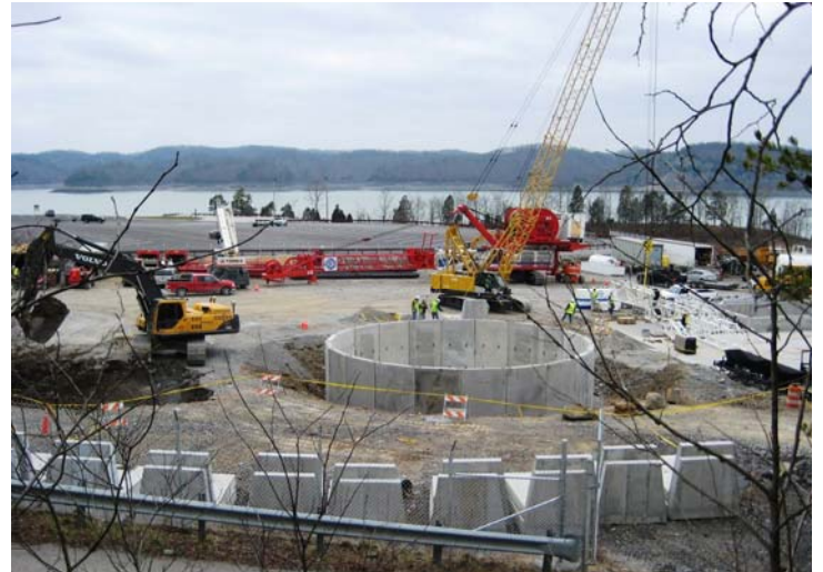
Staging area activity at Halcomb's Landing includes equipment assembly, and installation of desanding units, slurry ponds, and water silos.
